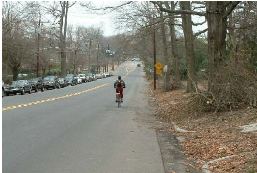
Figure 8. This 22 foot lane results in debris reducing the usable width. Cameron Avenue, Chapel Hill, NC.
